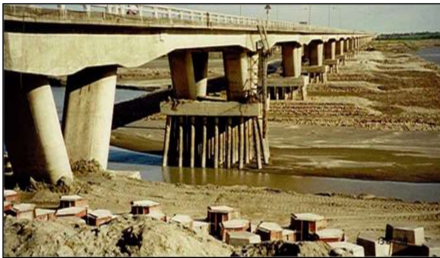
Fig.1 Local scour around the foundation bridge
